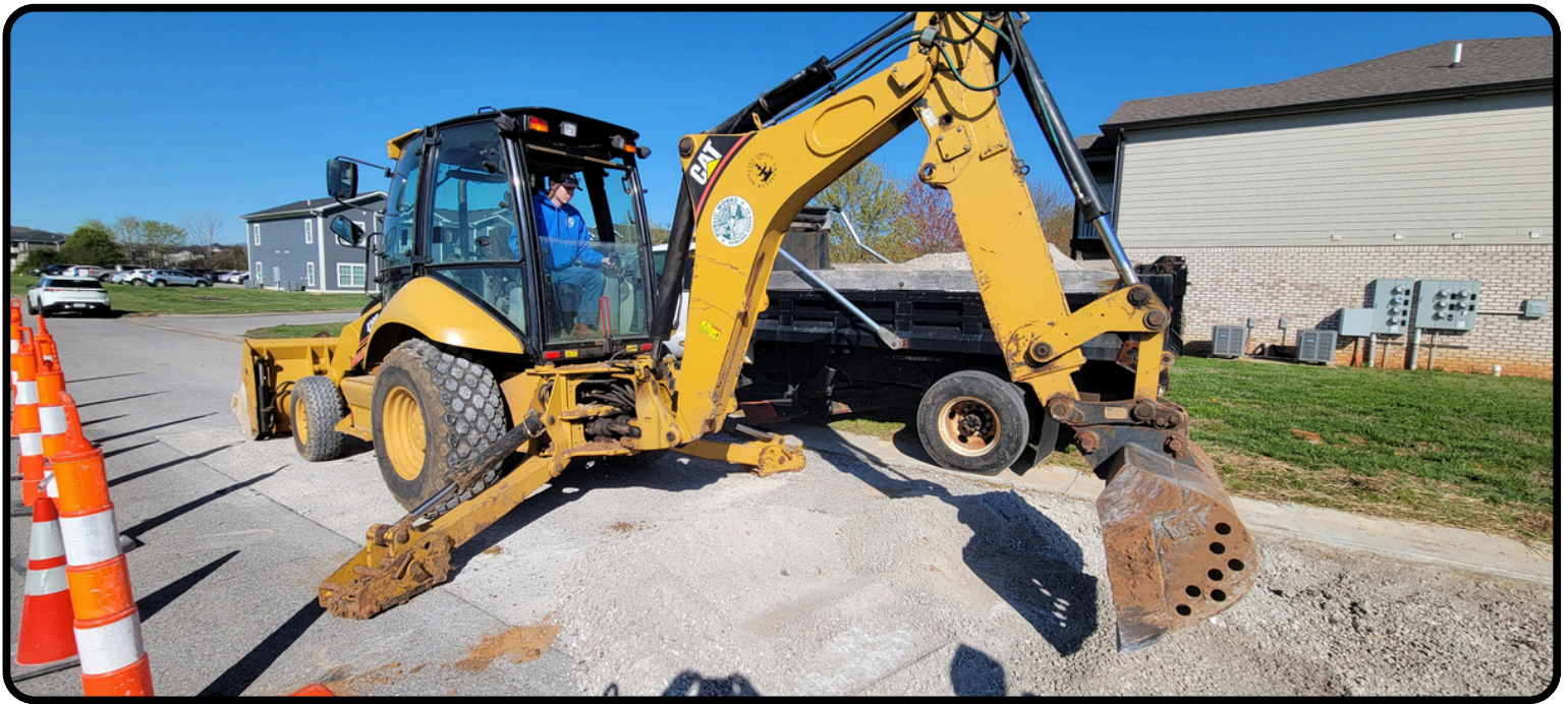
Operations Maintenance Technician I Jacob Lyons prepares the roadway for a sinkhole repair on Worth Way , near Russellville Road/US Rte 68 (24 March)
