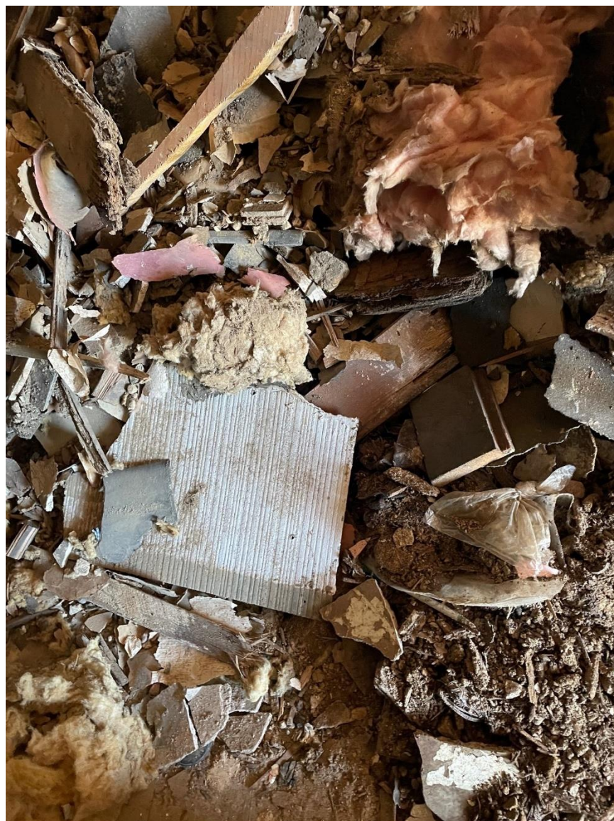
Photo 3. Asbestos containing transite panels. Location: Dining Room debris pile
