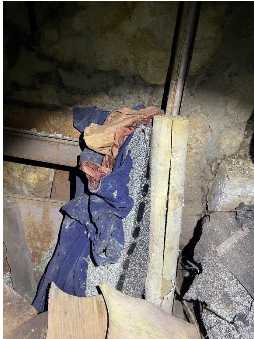
Photo 1. Pipe Insulation Debris. Location: Basement next to the exterior door
