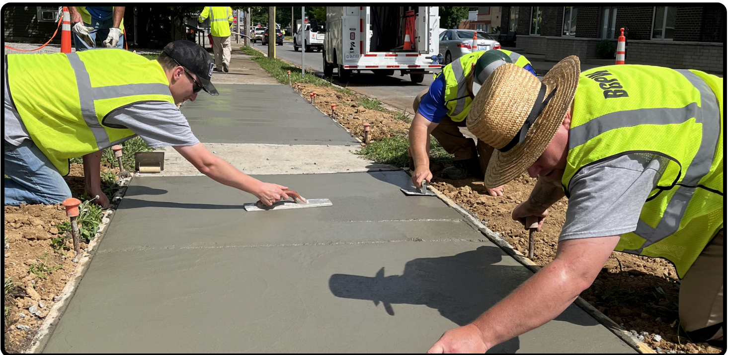
The operations crew addressed tripping hazards near East 6th Avenue and Chestnut Street (May 28).
