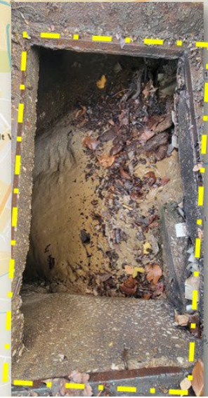
Flowstone buildup in the Whiskey Run storm drain
