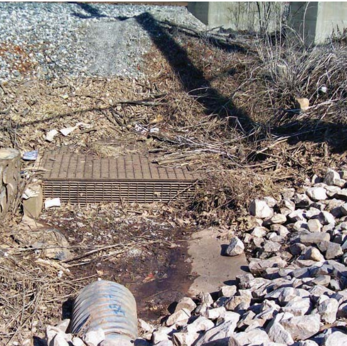
Sediment and debris impacting drainage well
