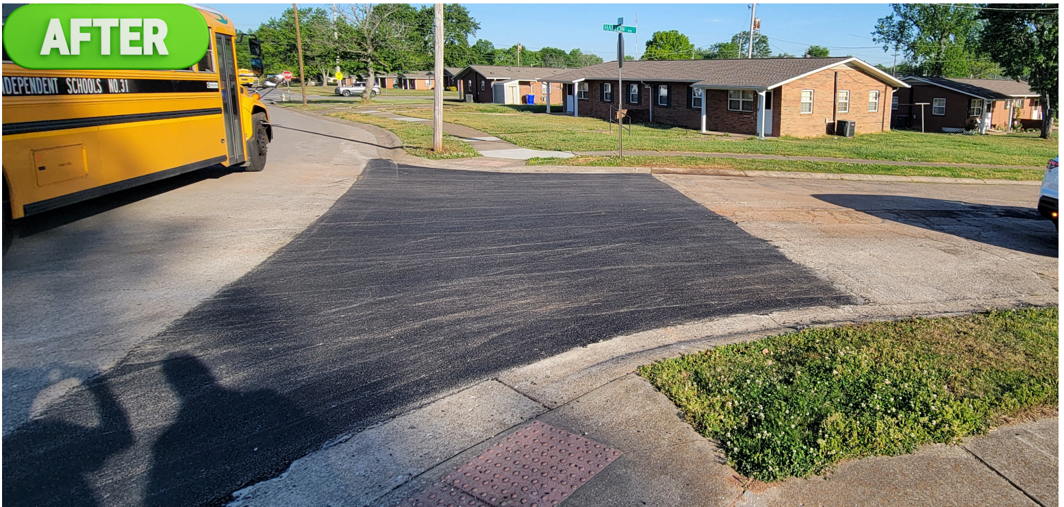
Operations crews repaired deteriorated pavement at Scott Way & Harlow Way , restoring safe ADA ramp access. (Month of April)
