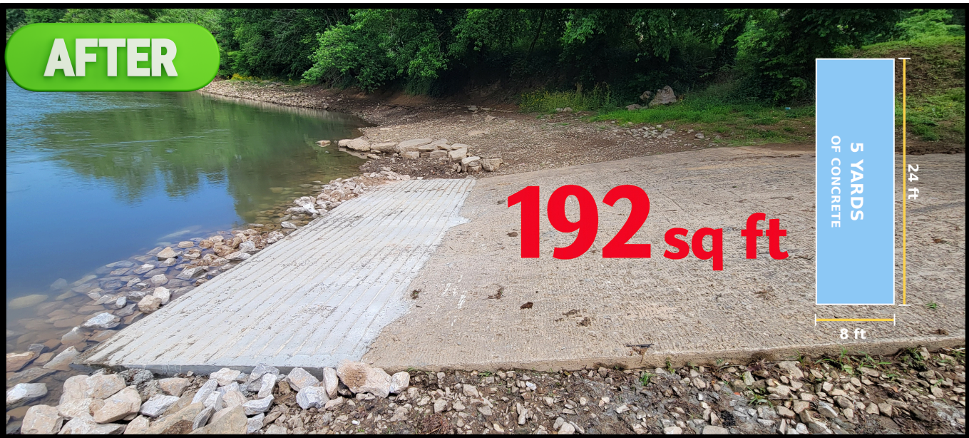
The Public Works crews utilized the dry weather and low river levels from April 24 to 27 to extend the boat ramp and add new signage on Boatlanding Road .
