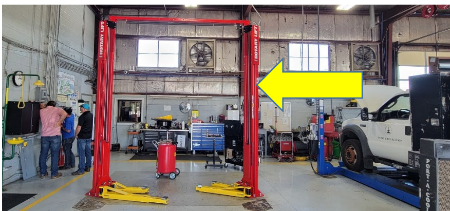
Figure 10-Facilities Technicians Caleb Houtchen and Kenny Woods troubleshoot an electrical issue with a newly installed lift at Fleet Division (27 June)
