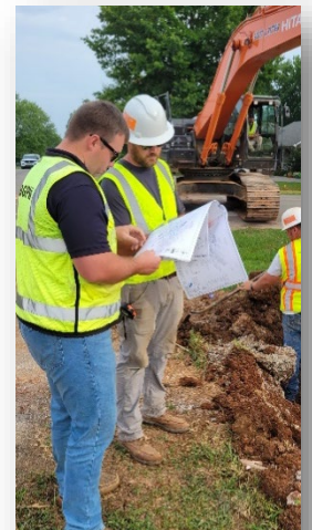
Figure 6-Construction Coordinator II Tyler Phelps reviews plans during the construction of the Westen St/Highland Way roundabout (18 June)
