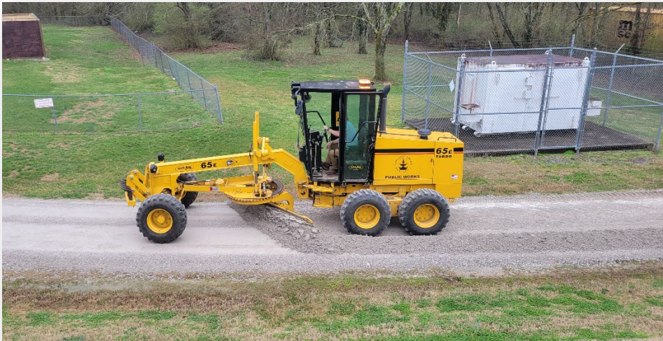
Figure 2- Operations Maintenance Technician II Doug Hoots grades the road at the Bowling Green Police Department Shooting Complex (7 March)
