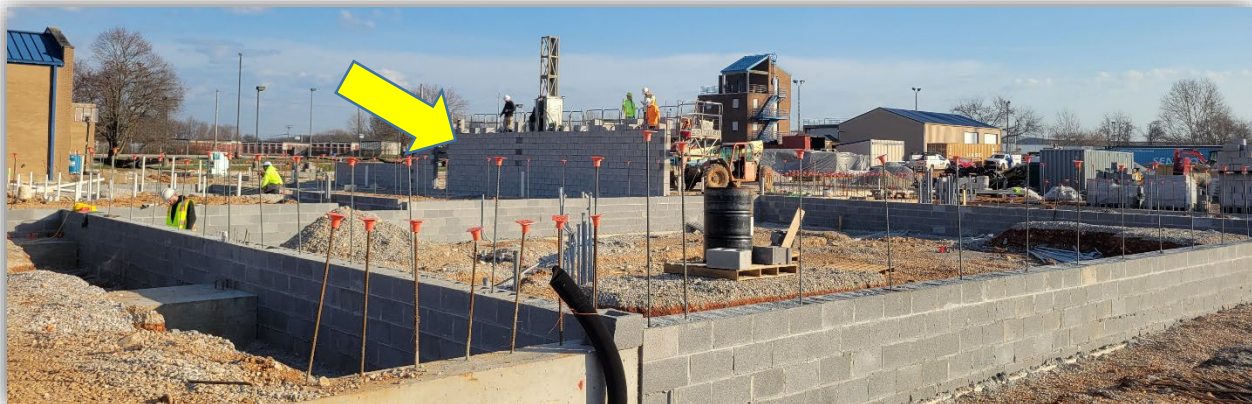
Figure 12-First walls going up at the Public Safety Training Center on Porter Pike (14 March)
