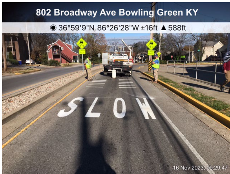
Figure 4- Operations crews install rumble strip markings at Broadway Ave & High Street to help improve safety after multiple speeding accidents this year (16 Nov)
