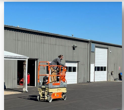
Figure 8- Maintenance Technician Caleb Houtchen prepares to service lighting at Fleet (2 Nov)
